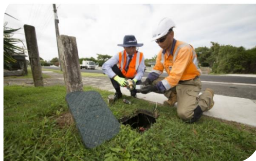
Figure 30: Checking a water meter. Credit: Watercare
